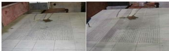
Figure 7. Damage incurred on impact side of ECC100 panel, A) after the first impact, B) after the 10 th impact
